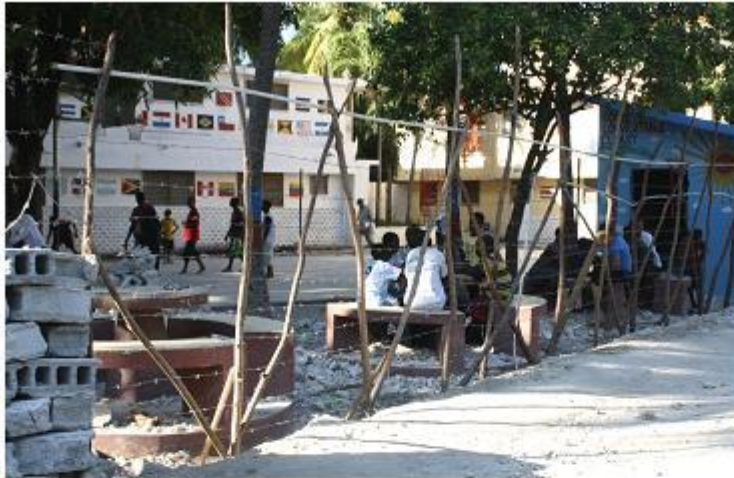
Continuing with recovery efforts, we removed two hazardous wall sections and replaced them with temporary fences. This removes hazard while maintaining the perimeter for security purposes. Cement wall construction will begin next week.
